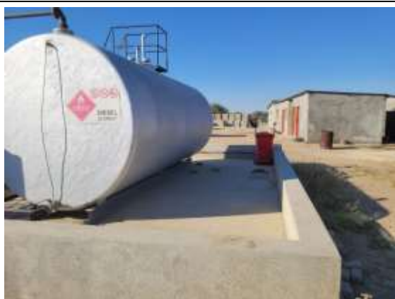
Photo 4-1 Existing storage tank inside a bund wall
