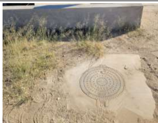
Photo 4-4 Oil water separator
